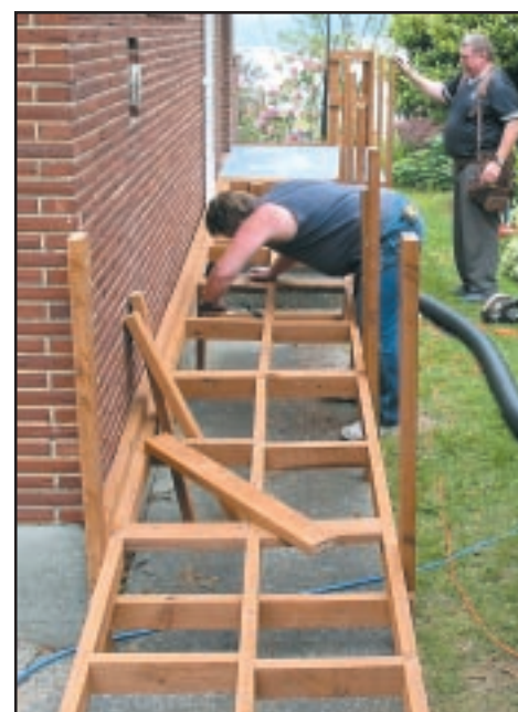
Photo right: Vennie Murphy and Phil Hicks build the framework for a ramp.
