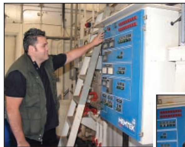
Above: Jim Absolor serves as the Waste Water Treatment Operator at Boeing Electronics Center.
